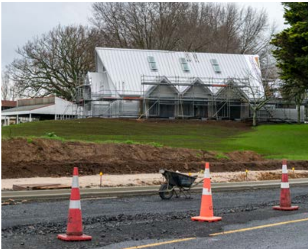
Work continues on the chapel and roundabout at the Paeroa Hills development.
