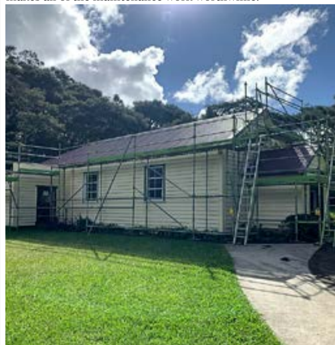
Kauaeranga Valley Hall under scaffolding during recent roof restoration and maintenance work. Photo: SUPPLIED
