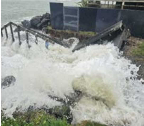
Damage to Iti Lane beach access, Cooks Beach. Photo: TCDC
