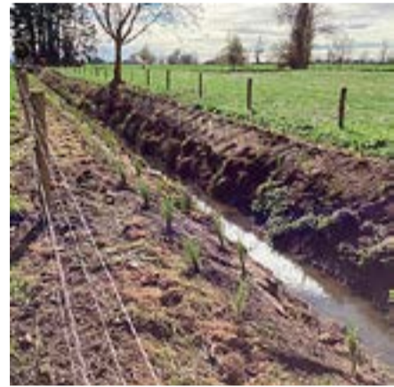
Johan van Ras says native sedges "are insane at holding the banks together". BELOW: A drain post-fencing and planting. Photo: SUPPLIED
