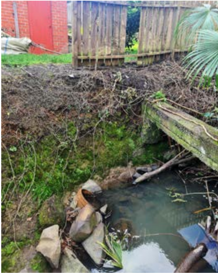
The culvert behind Chris Kemp’s property is eroding the bank. He has been trying to get it fixed since December. Photo: SUPPLIED
