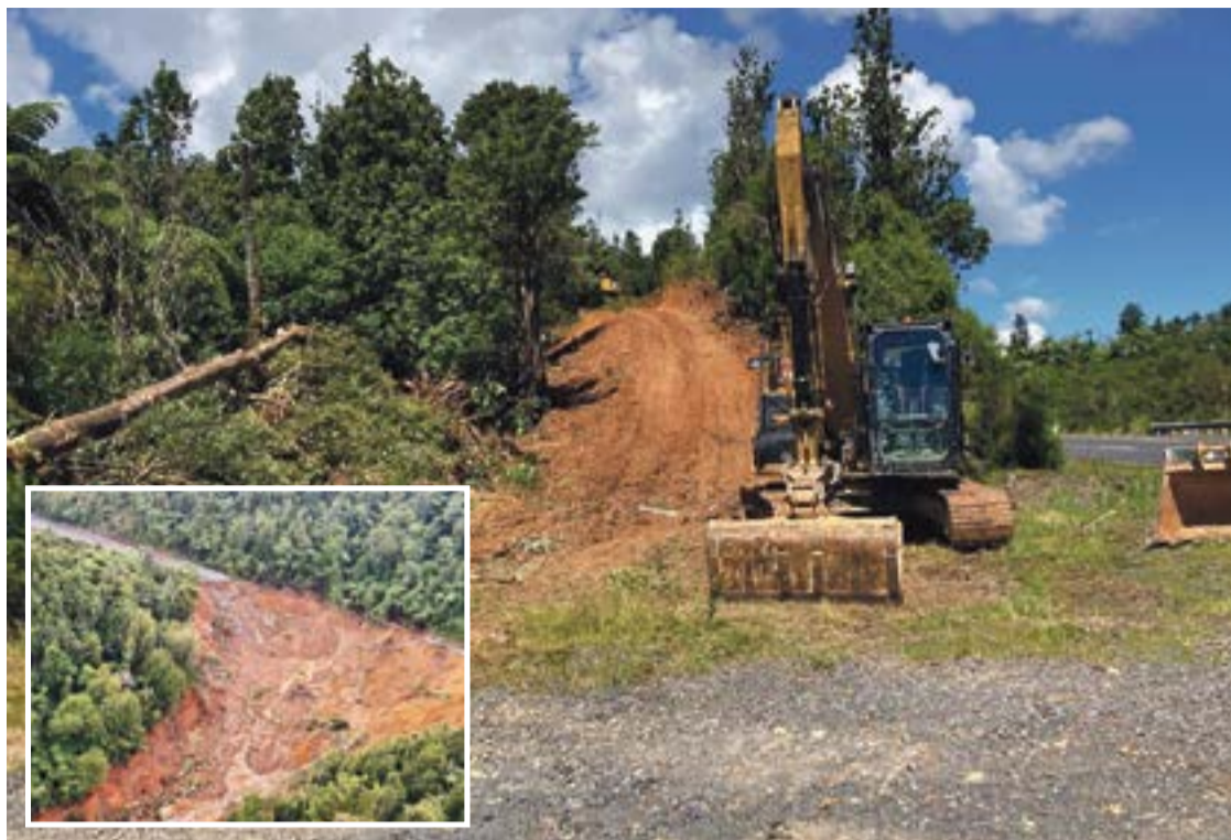
An access track is being built for geotechnical drilling rigs at the slip site. INSET: The missing section of road.
