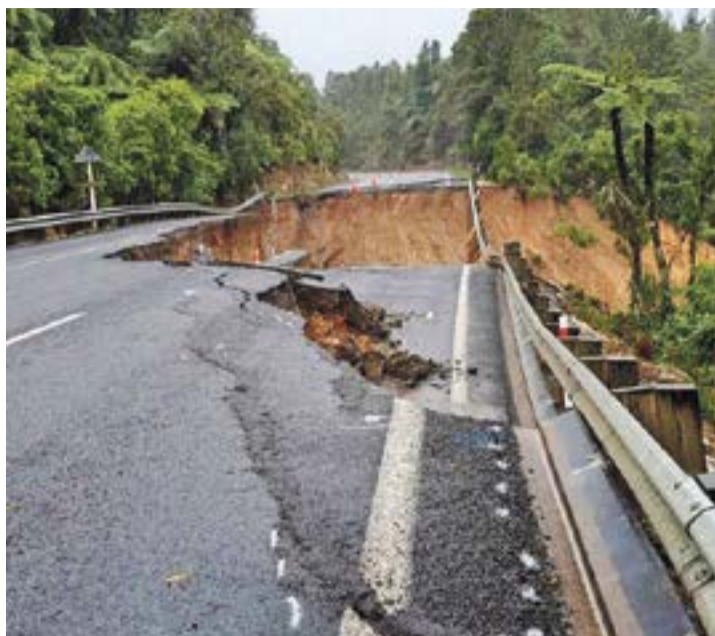
SH25A collapsed further over the weekend.
