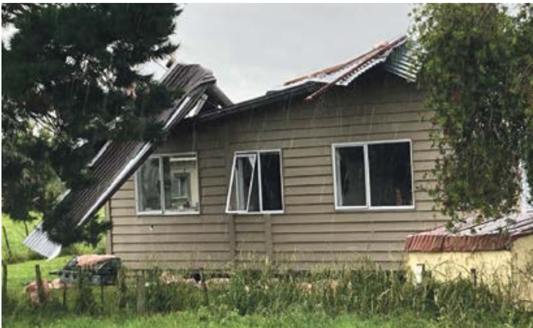
A rural home near Kerepēhi lost its roof during the storm.
