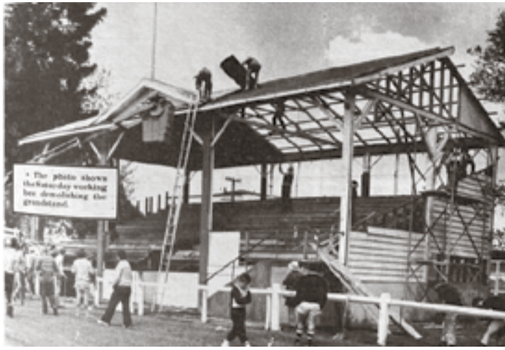
Volunteers demolish the original grandstand in the Paeroa Domain after it was found to be unsafe. Photo: SUPPLIED
