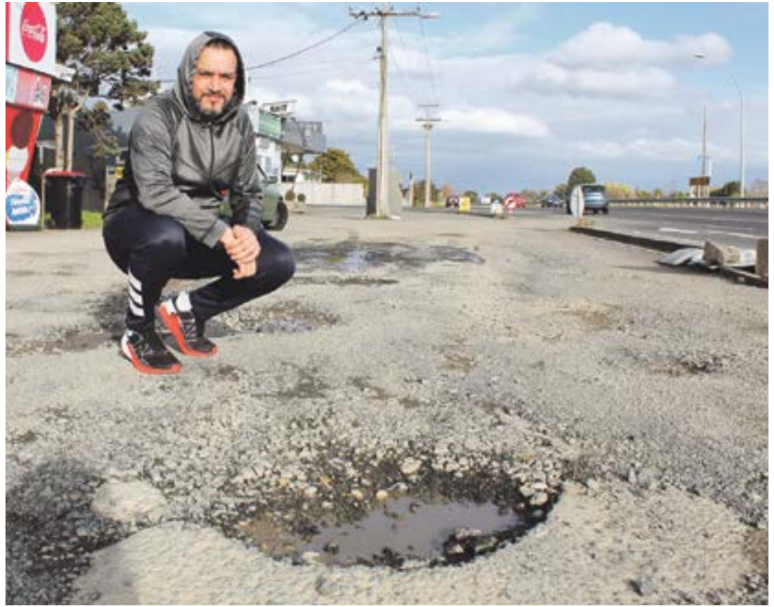
Harvinder Singh, the tenant of the Totara Superette, recently spent more than $1000 on pothole repairs.
