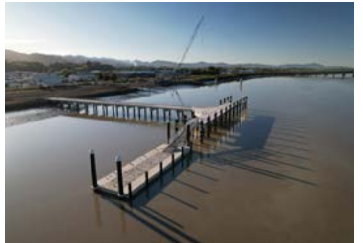
Work on the Kōpū Marine Servicing and Business Precinct is coming along nicely, in time for its opening in May. Photo: URBAN SOLUTIONS
