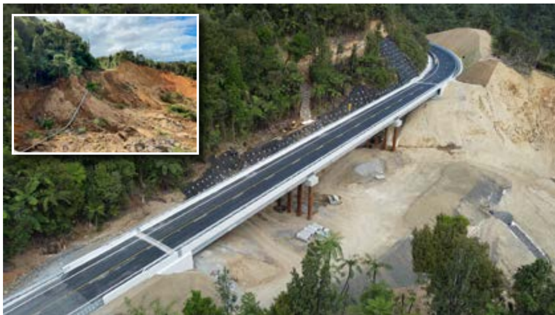
The new Taparahi Bridge on SH25A. INSET: The initial slip in February 2023 took out 110m of road. Photos: SUPPLIED
