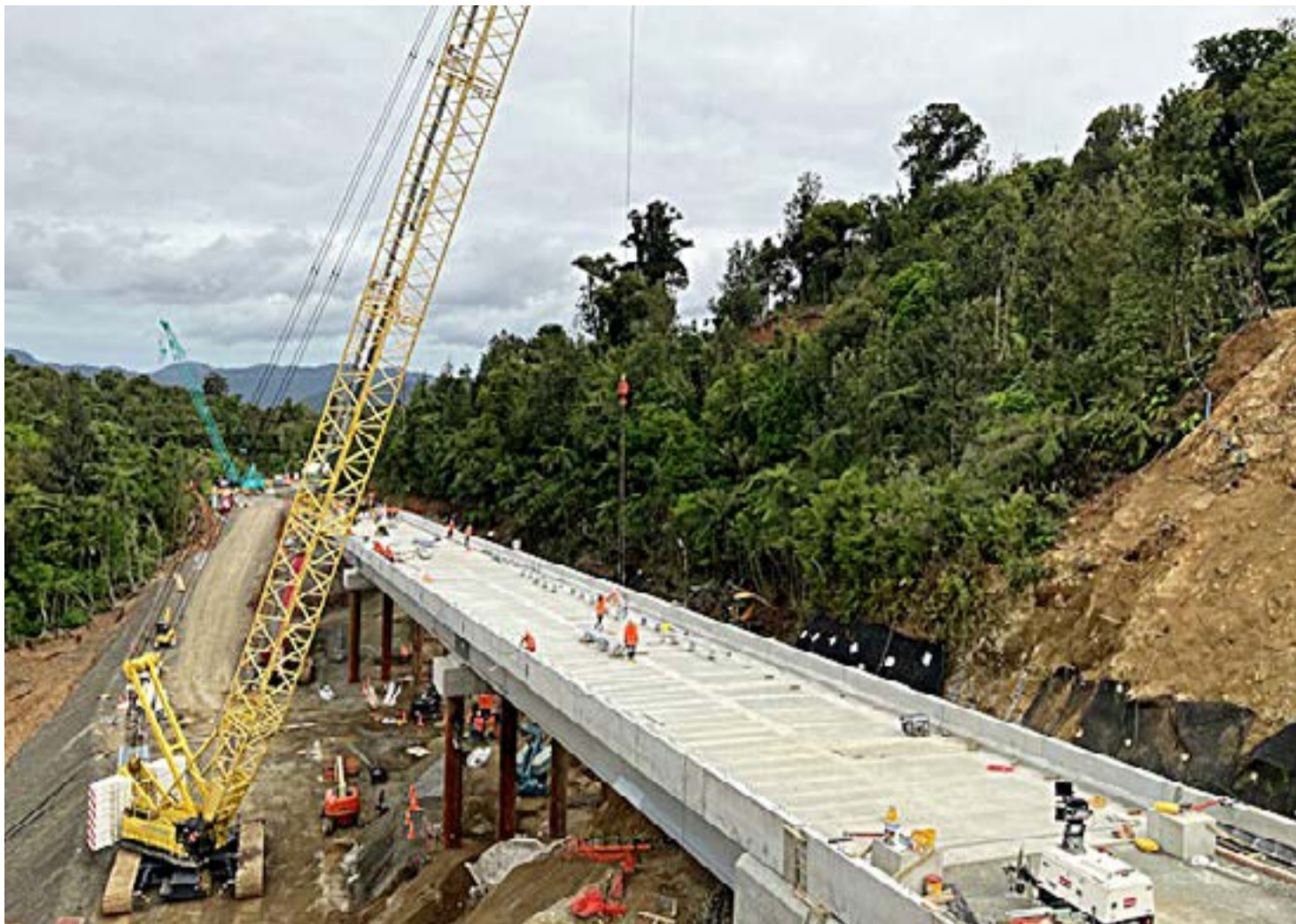
The latest photo of the 124m SH25A bridge on December 1 shows it is nearing completion.
