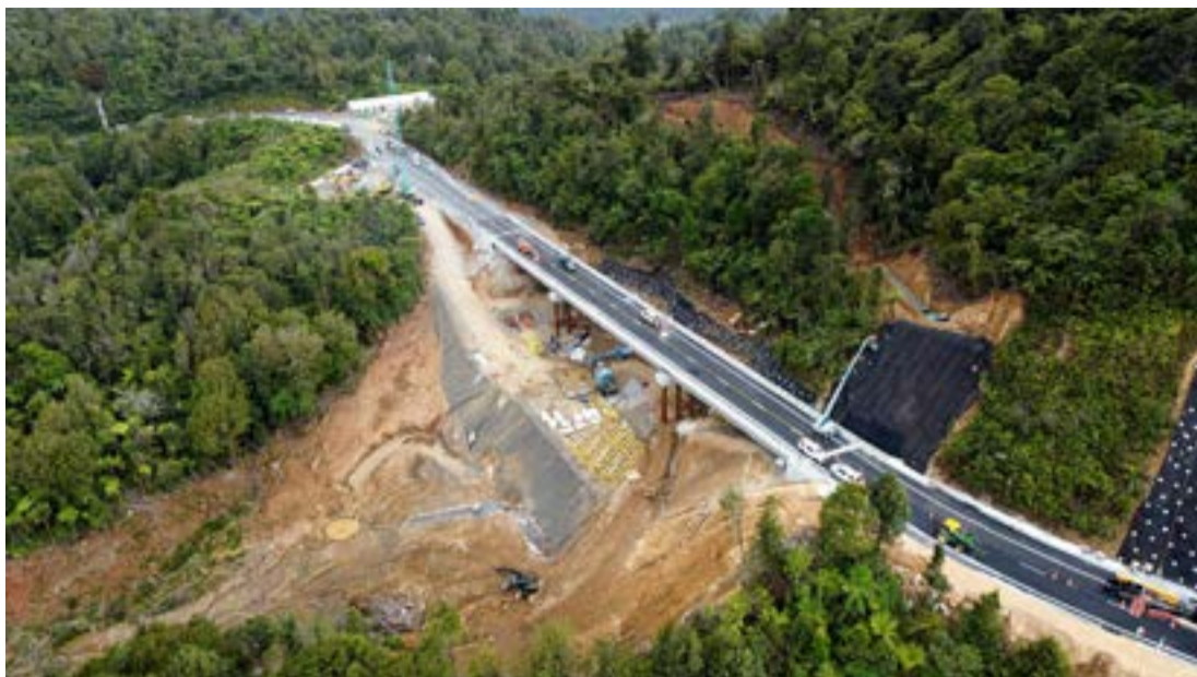
The now-completed Taparahi Bridge along State Highway 25A, as seen from above.
