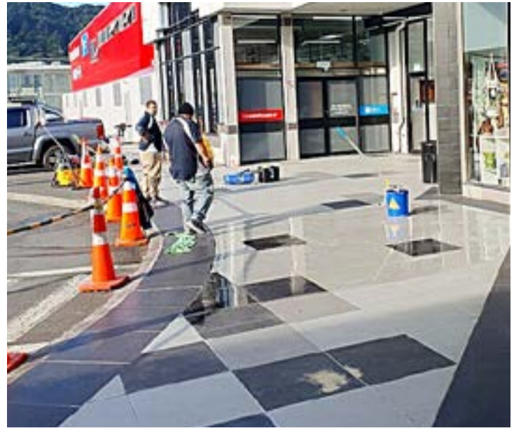
The exterior tiles have had a new anti-slip surface placed on top of them.
