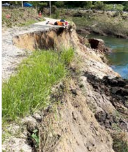
They Hauraki Rail Trail was badly damaged during storms earlier this year. Photo: SUPPLIED
