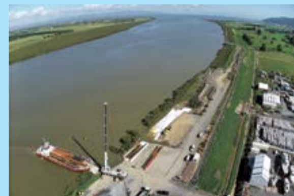
The first stage of road works, infrastructure and the base for parking and commercial areas finished in March 2023.
