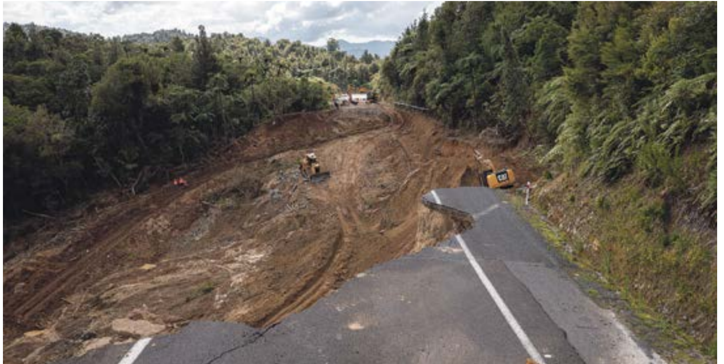
Work has begun on the gaping chasm on the road between Kōpū and Hikuai, but it's not an immediate fix.
